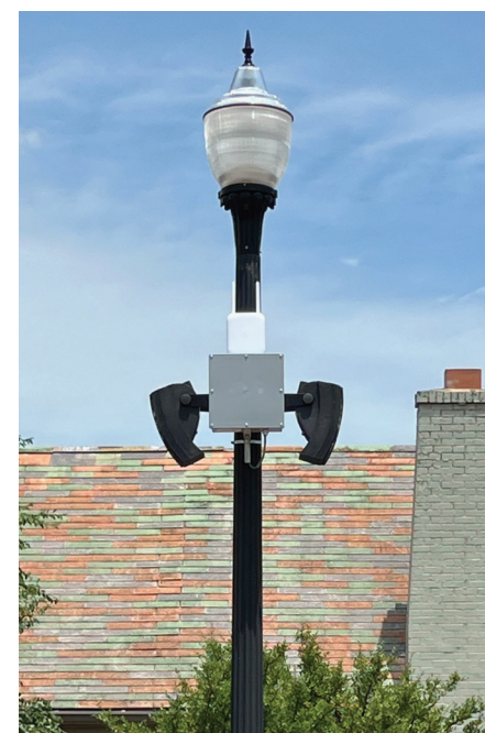
Exposed Speaker Station with WIFI-Reinforced Antenna
